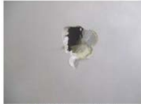
Figure 1: Damaged Gypsum Panel
