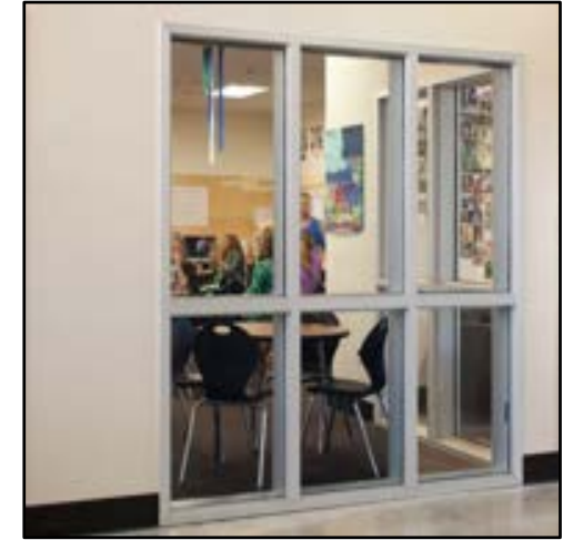
Interior Fire Windows
