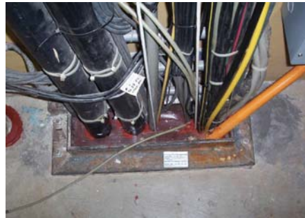
Proper firestopping is a team sport, specialty firestop contractor and qualified inspector.
