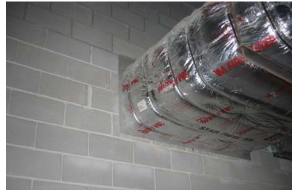
Stair pressurization duct is shown going through block.
