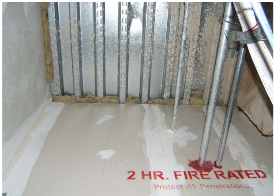
Compartmentation is penetrated by service piping. Ratings are restored using firestopping, fire dampers, fire doors and fire glass.
