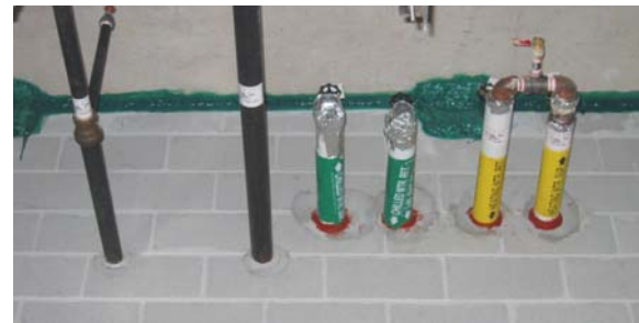
Various pipes include insulated and metal pipe.
