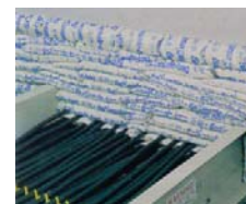
The quality process helps firestopping keep compartment sealed. (Photo courtesy of Grace Construction Products)
