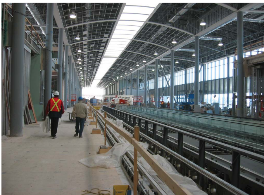
The Lester B. Pearson International Airport in Toronto is undergoing a C$ 4.4 billion project invested over 10 years.
