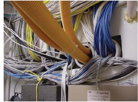
Contractor without quality process. Inadequate firestopping may result.
