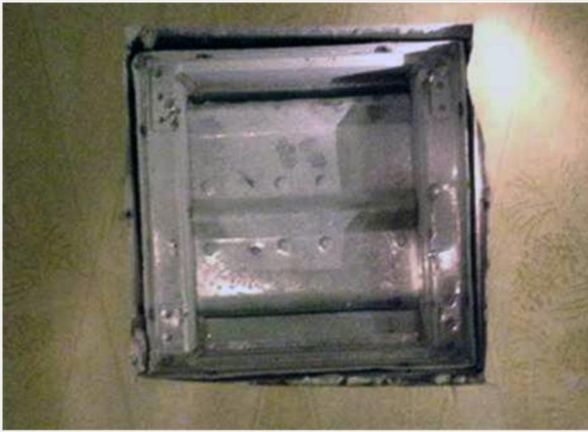
Damper installed racked.
