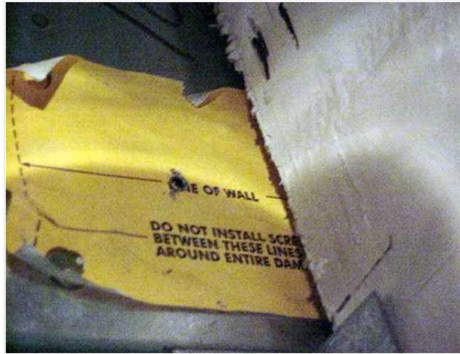
Screw fastened through linkage, through middle of warning label
