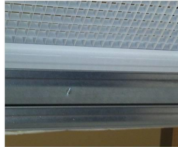
Screw fastened in track of curtain damper
