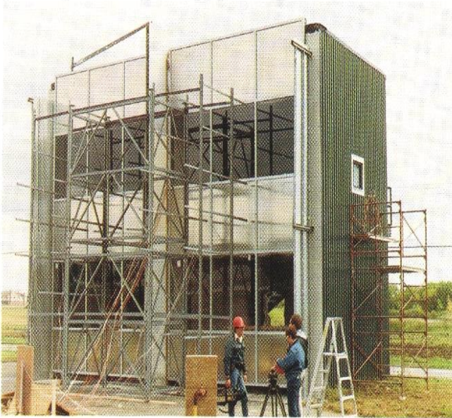
Fig. 1. Face of full-scale, permanent, fire-test facility at USG Corporation Research Center is set up for curtain wall fire test. Metal frame supports thermocouples for measuring flame plume temperature. Left side is "THERMAFIBER Curtain Wall Insulation Unit"; right side is "Glass Fiber Unit."
