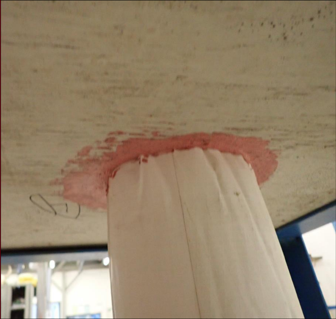
Pex insulated with fiber glass insulation
