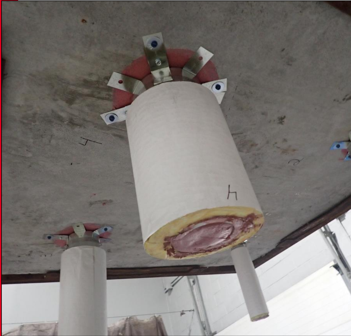
Pex insulated with fiber glass insulation with Firestop Collar
