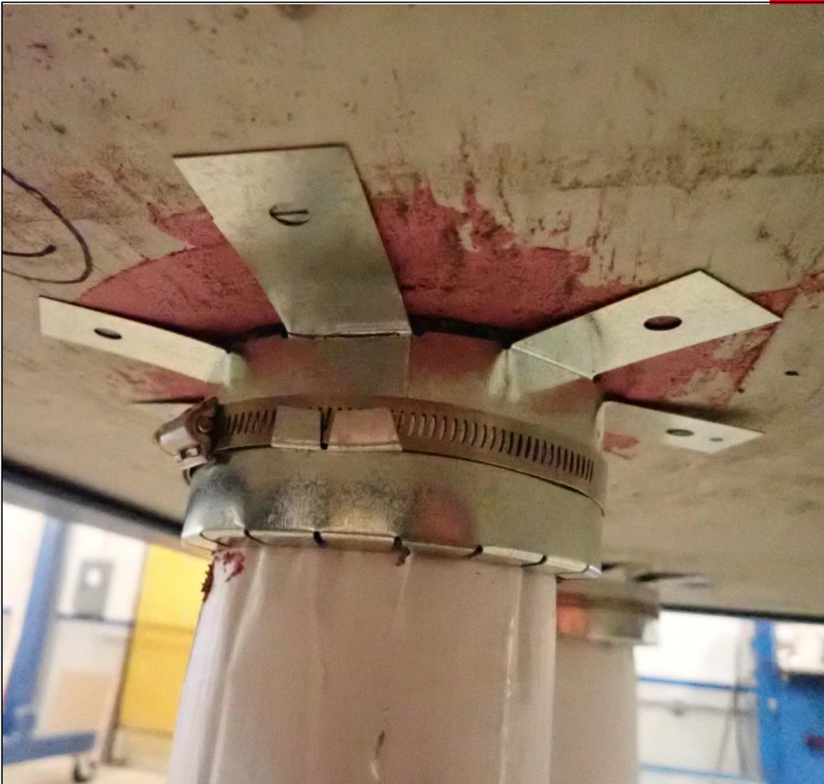
Firestop Collar installed around insulated Pex
