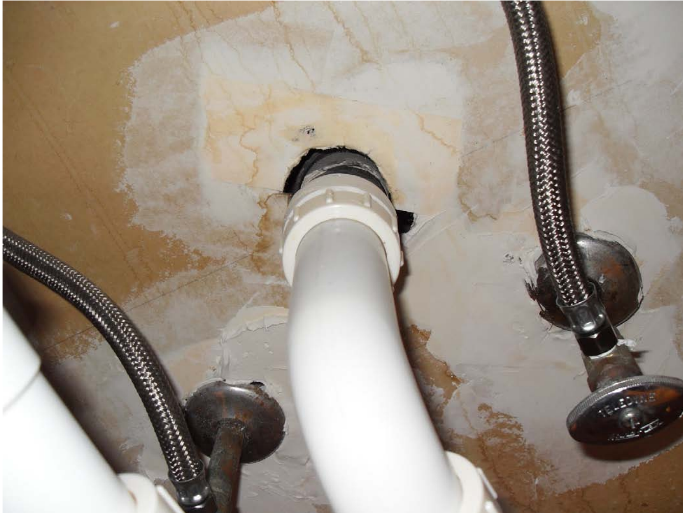
Firestop damaged around plumbing due to excess water leakage
