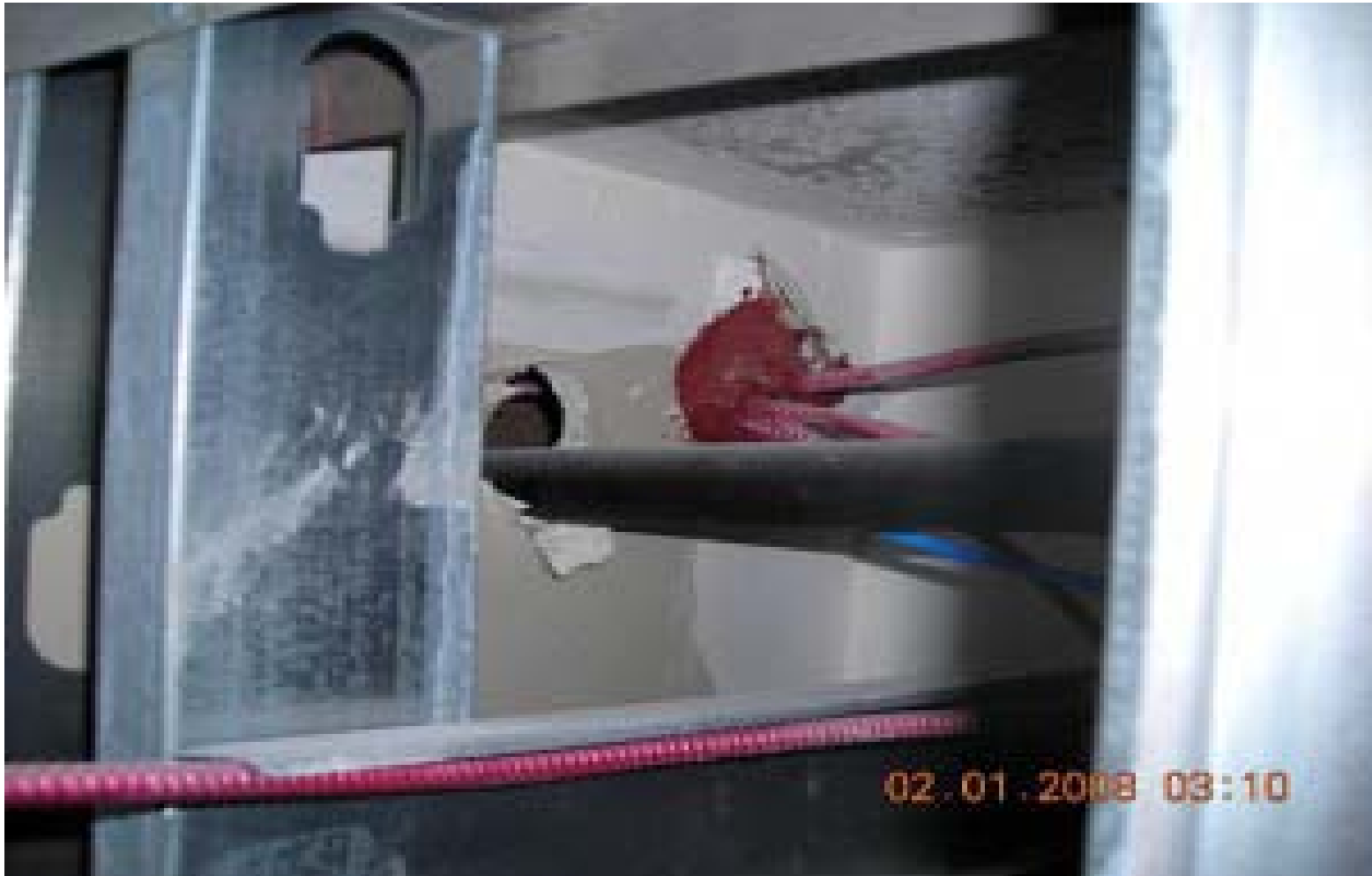
Firestop damaged due to pulling new cables in the electrical room
